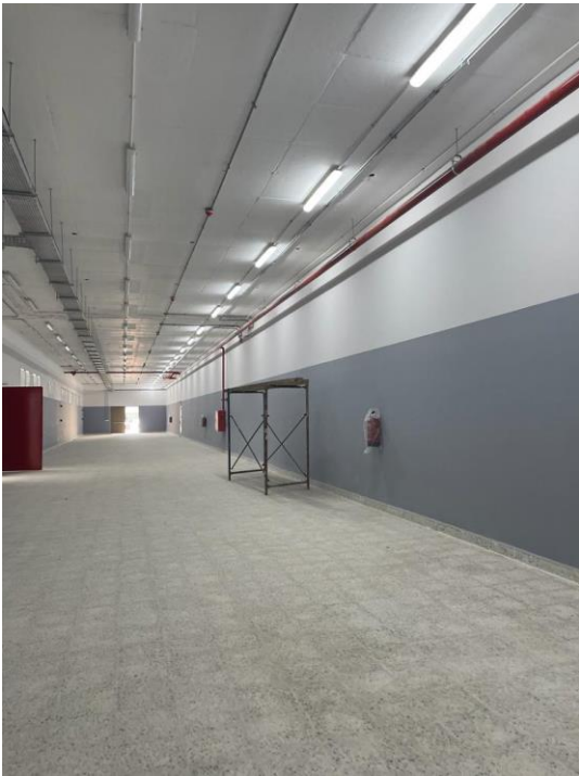
Figure 7: Empty workshop equipped with firefighting system and fire extinguisher.
